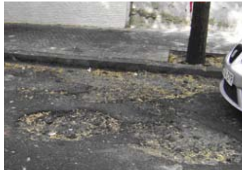
Figure 12: Distresses produced in an urban pavement by a car fire
